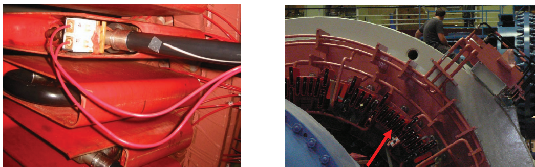
Fig 7: SFOAs mounted on the end winding connector of a 300 MVA generator
