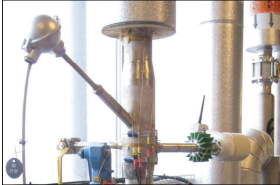
Figure 8 Pilot-installation of an autonomous and non-invasive temperature device, before insulation, close to a standard thermowell installation for benchmark purposes.
