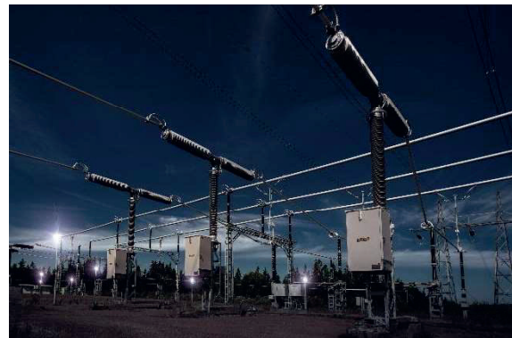
Fig. 1: High voltage circuit breakers in an electric power transmission substation with integrated fiber-optic current sensors [10].
