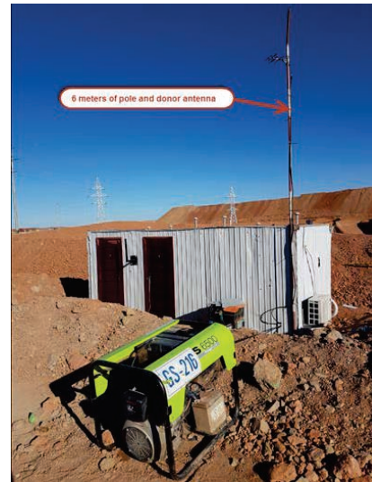
Fig. 9. RF donor antenna location
