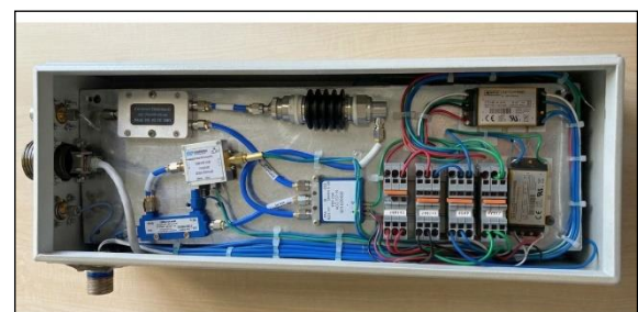
Fig. 2. Internal view of the RF protection control box showing the RF switches, power detector, relay modules, and wiring.
