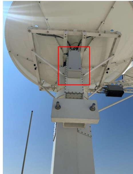
Fig. 5. The RF protection system control box installed on the antenna pedestal of the telemetry ground station.
