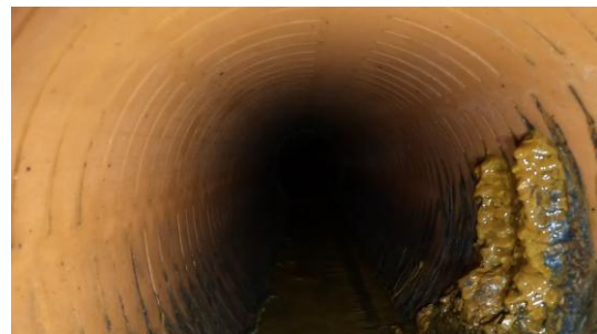
Figure 5: Strong scaling with reddish color at the side wall of the pipe
