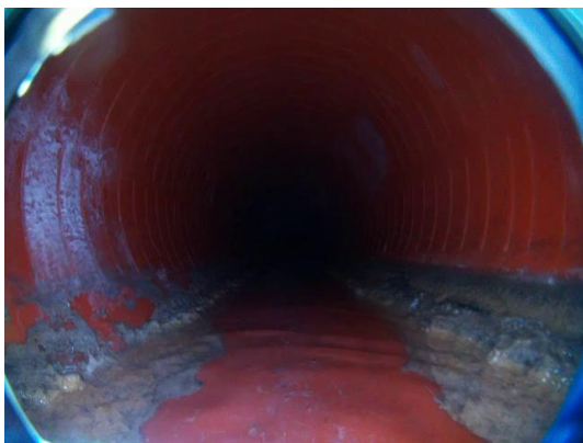
Figure 3: Medium to severe scaling at the bottom, slight scaling at the side wall
