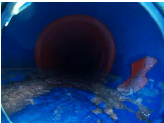
Figure 2: Medium to severe scaling, visible hole in the pipe wall
