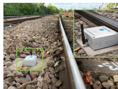
Fig. 1. Wireless tiltmeter installed on a railway sleeper for real-time track monitoring.
